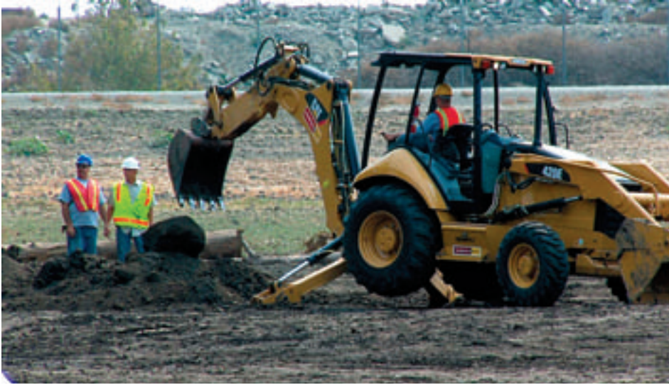
Part of the instruction focuses on operating equipment smoothly and efficiently. "We work on the ability to be very precise," says Chris Cannon. "If you're digging a footing as opposed to a basic trench, your tolerances are a lot closer, and you have to be able to dig those back walls."
